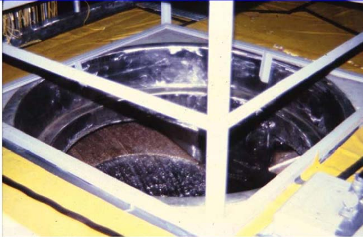
Skimmer Surge Tank
